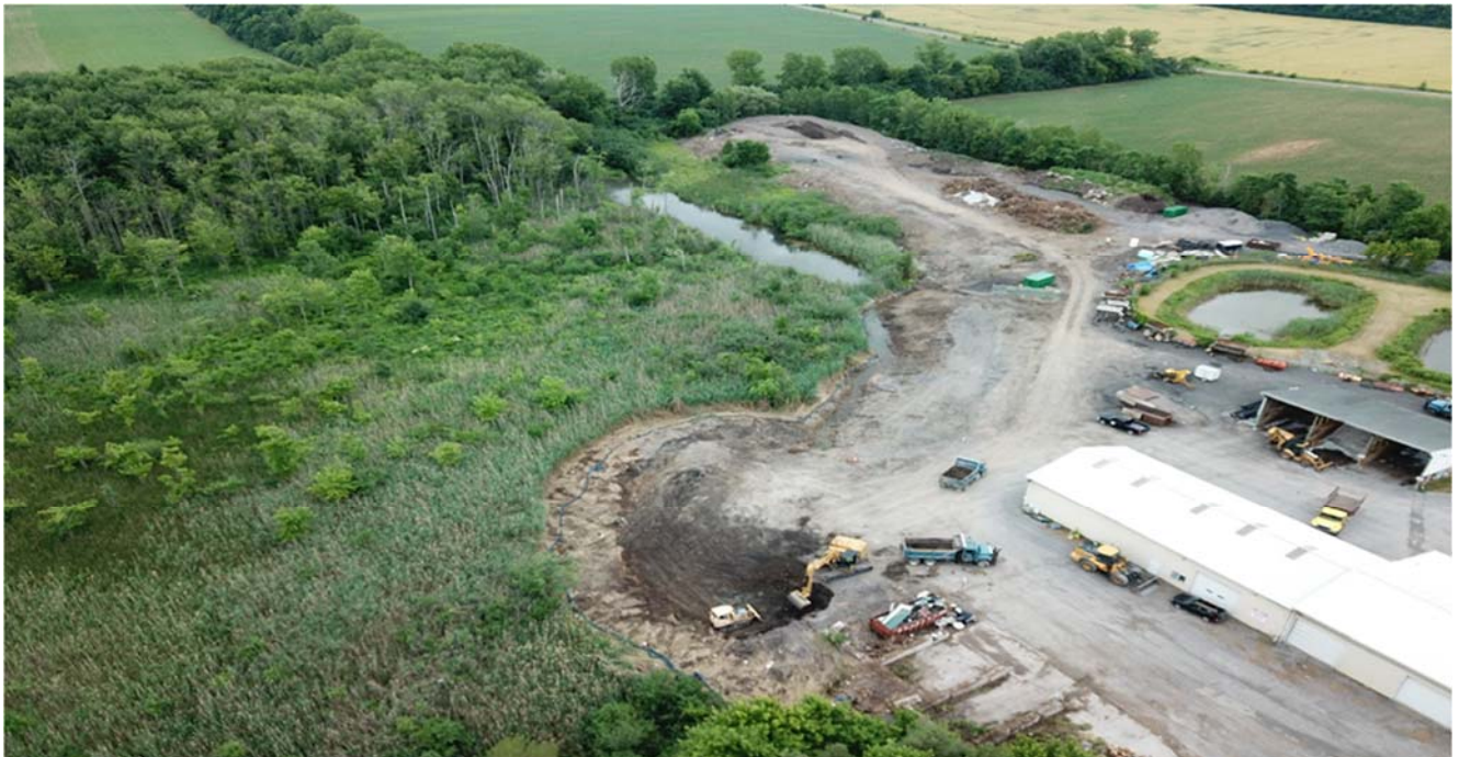
An overhead view of the Owasco Public Works wetland restoration area. Excavation of new wetland area began in 2020, illustrated in the center of the photo.
