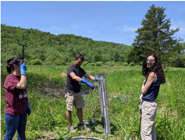
Drew Snell, Ally Berry and Tehya Kloster add a stop log to the water control structure
