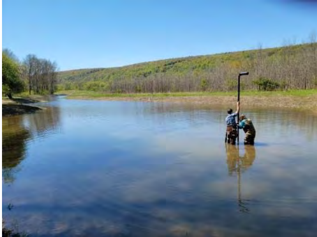
Michele Wunderlich and Drew Snell install a Hyfi Sensor in Basin #3. Photo by Ally Berry.
