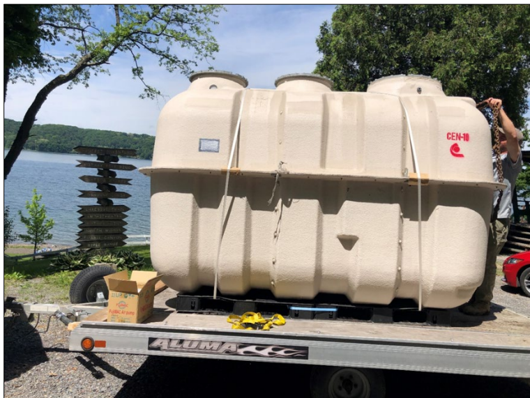
Photo (credit: Olivia Green): The nitrogen-treating FujiClean CEN 10 system awaiting to be installed at the Auburn YMCA's Camp Y-Owasco along the Owasco Lake Shoreline. A passive phosphorous filter follows this system in the "treatment train", followed by a new leachfield.
